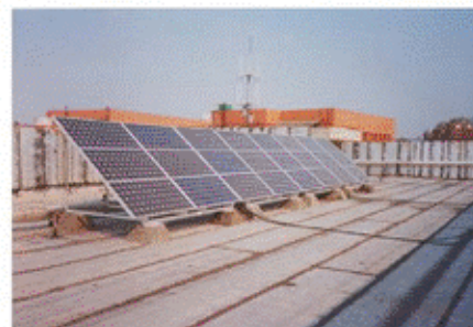
Jiangsu provincial party committee yard solar power station project
