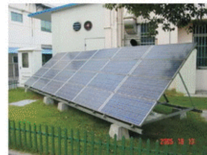
Shangde factory area solar power station project
