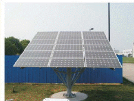
Suzhou aimosheng committee yard solar power station project
