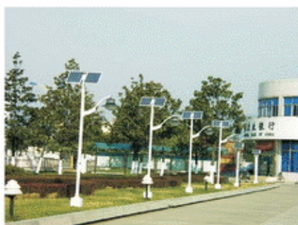
Wuxi city lihu garden country club lighting project
